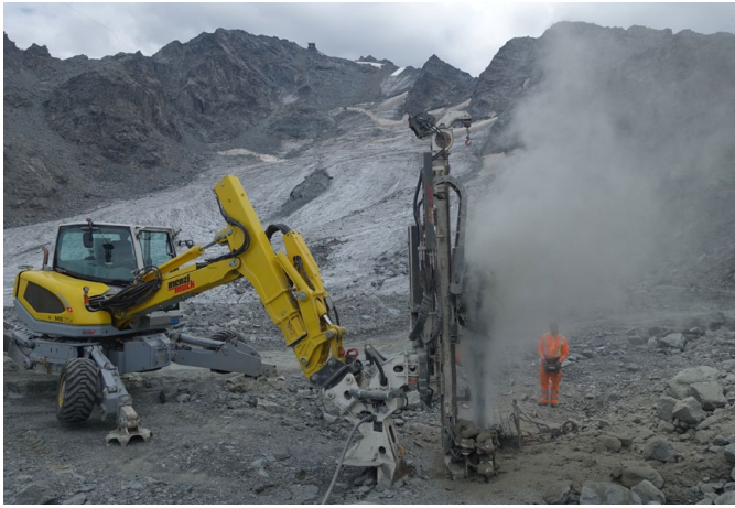
Fig 64. Drilling a new borehole in the frozen moraine at Gentianes (2022) to secure the 20-year permafrost temperature time series. Photo: Christophe Lambiel.
