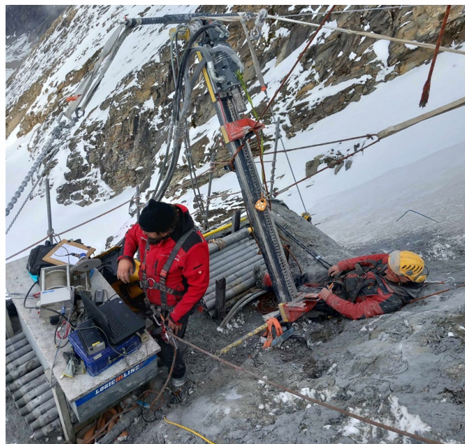
Fig. 8. Deep boreholes (20-40 m) being drilled and equipped with inclinometers and thermistors at the OpAL site, Kitzsteinhorn, Hohe Tauern Range. Photo: Ingo Hartmeyer.
