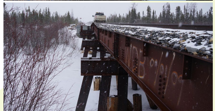
Fig. 14. Gunghi Creek survey (top; photo: Nick Kozachuk) and Hudson's Bay Rail bridge frost heave effects on piles (bottom; photo: Natalie Arpin).
