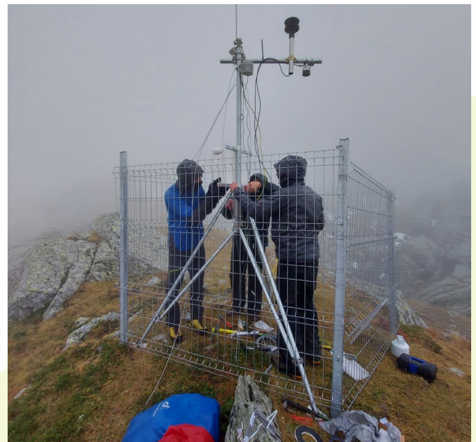
Fig. 54. Installation of the automatic Campbell Scientific meteorological station on Căldarea Pietroasă cirque. Photo: Alexandru Onaca.
